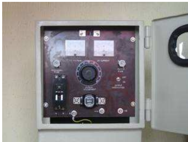
Front view of rectifier with door open showing the output control knob, meters, breaker, Switches, surge suppressors, input and output terminals and fuses.
