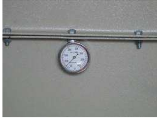
Side view of rectifier showing the oil temperature gauge (Thermometer)
